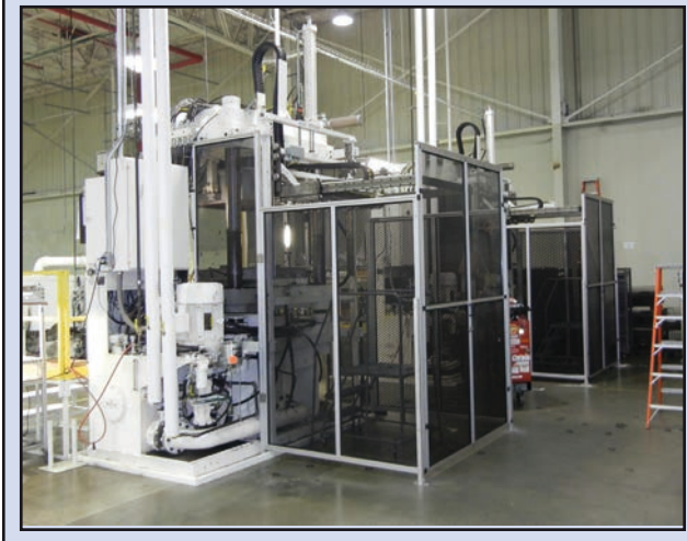
Figure 3 - interlocked guarding around the presses protects employees during operation
